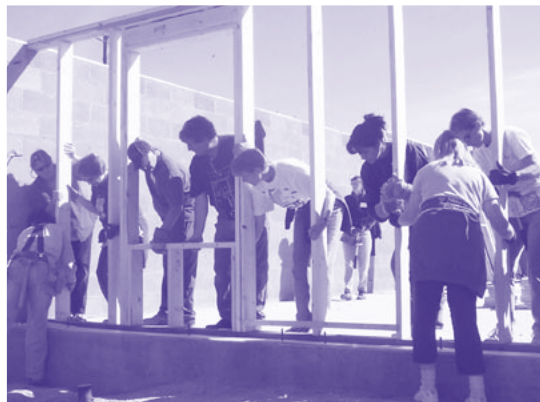
Volunteers raise the first wall at the Habitat for Humanity Rainbow Build
